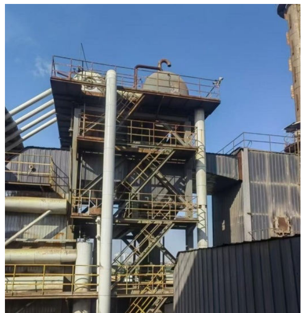
Photo: Biomass boiler equipped with environmental protection facilities. Source: China Chamber of Commerce for Import & Export of Light Industrial Products & Arts Crafts, 2024
